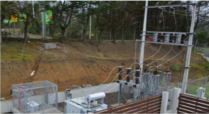
Fig. 3. Power conversion center.
